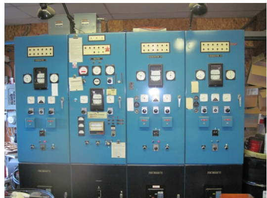
Figure 1 Current switch gear (37 years old)
